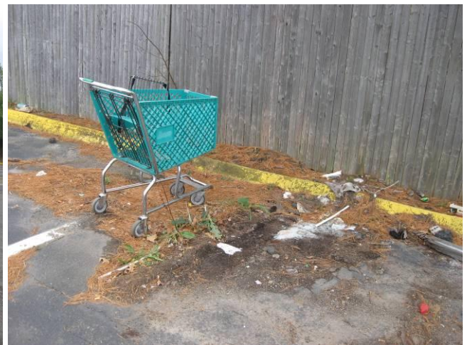
The parking lot pavement is breaking up and stained and sediment and debris have collected in some areas.
