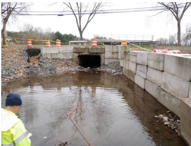
NBP-19: Channel heavily and recently modified upstream of Burnham Street.
